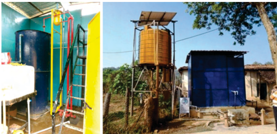
Figure 68: Self-Sustained Auto Backwash Iron Removal Plant
