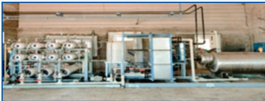
Forward Osmosis system installed at Narippaiyur Village
