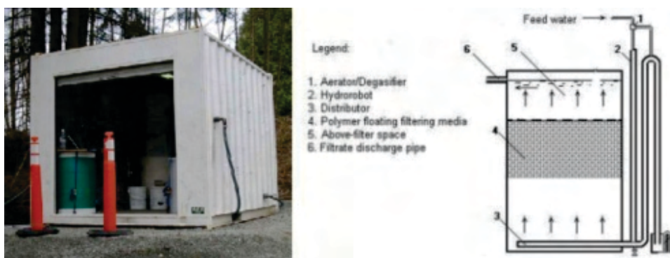
Figure 67: Iron Stopper Containerized Treatment System
