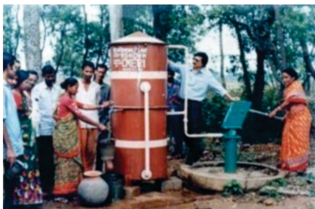
Figure 56: CMERI Iron Removal Plant
