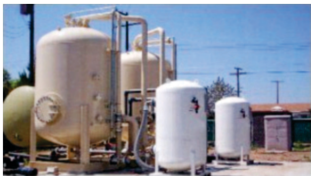
Figure 73: Siemens Nitrate Removal System
