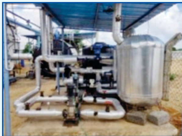
Solar hot water system installed
