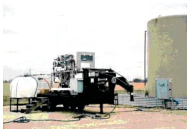
Figure 91: A&M Mobile Desalination Unit
