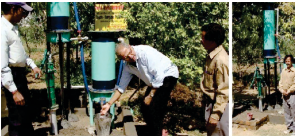
Figure 34: Arsenic Removal Plant at Rampur - Maner
