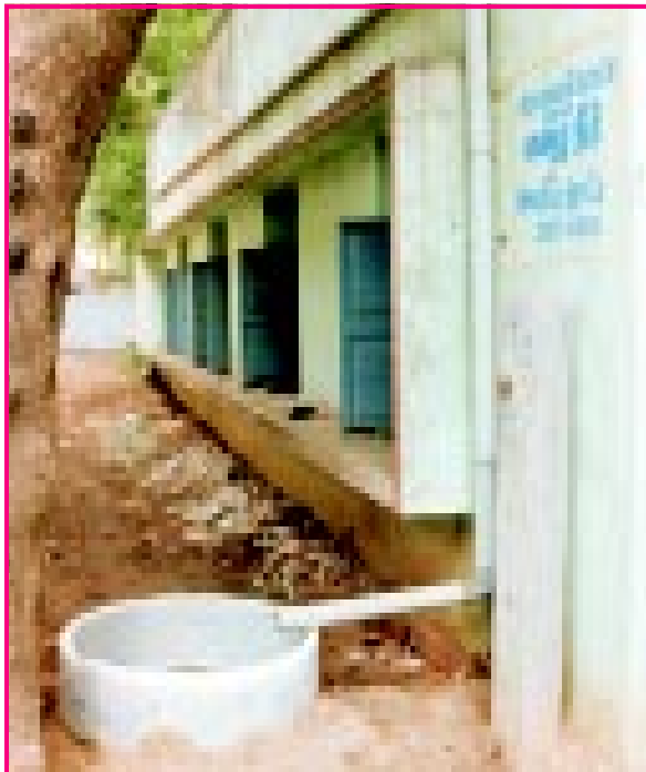
RWH in Panchayat building
