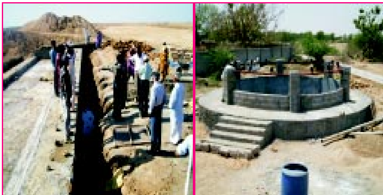
NALIYA DRINKING WATER SCHEME
