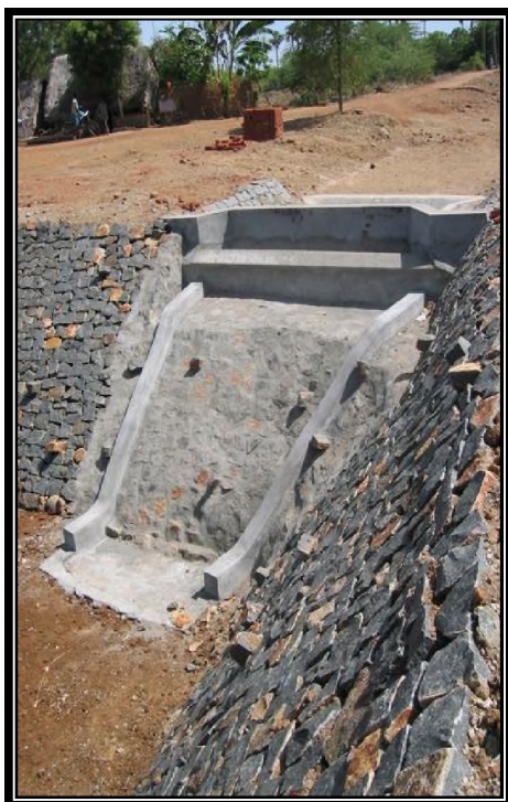
8.19 (a) Settling Basin
