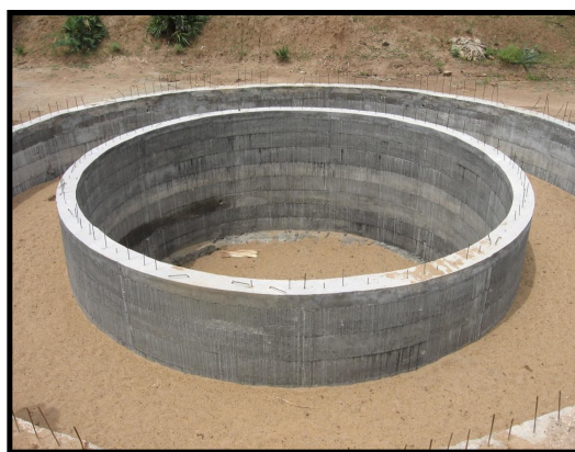
Recharge Shaft in namakkal District in Tamilnadu
